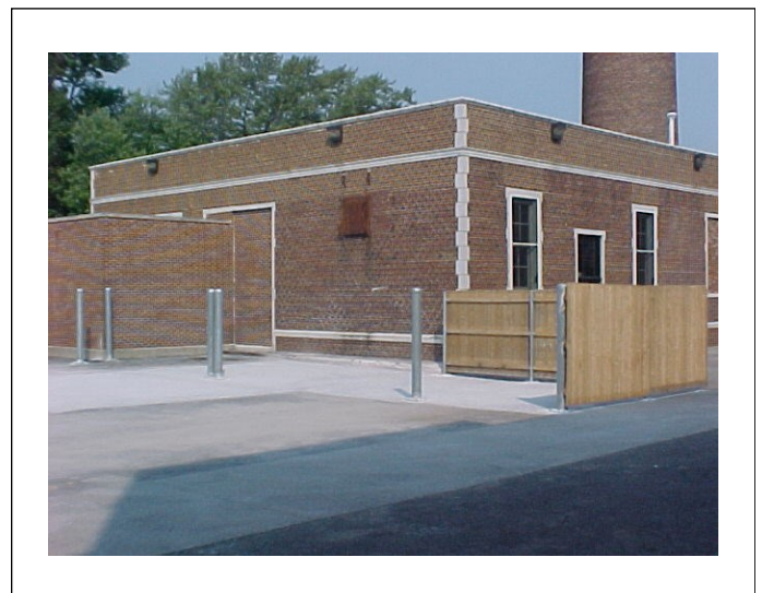
Final construction nears completion in the dumpster and parking lot areas of the school.
